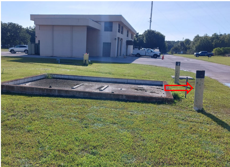
Photo 4 – LBP yellow metal parking bollards on Structure 5
