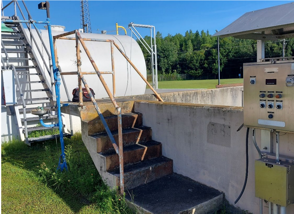
Photo 3 – LBP orange metal handrail on Structure 3
