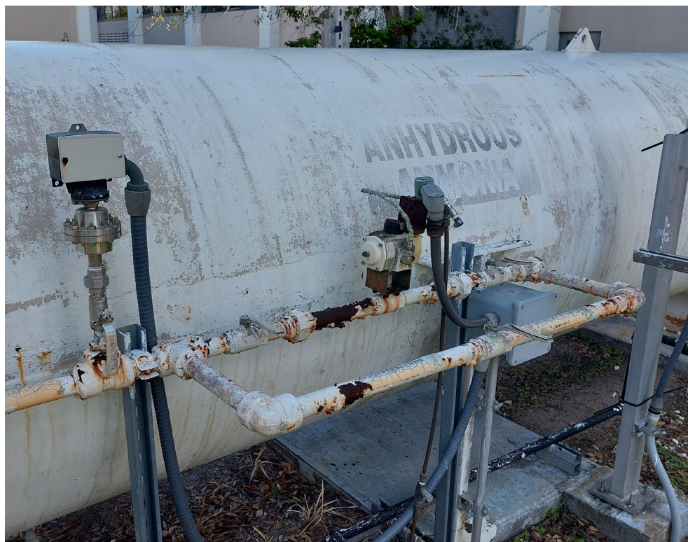
Photo 22 – “Chlorine Tank” labeled “Anhydrous Ammonia” in field
