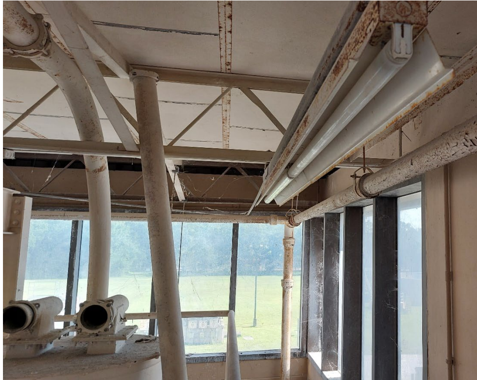
Photo 15 – Fluorescent light fixture with four-foot bulb
