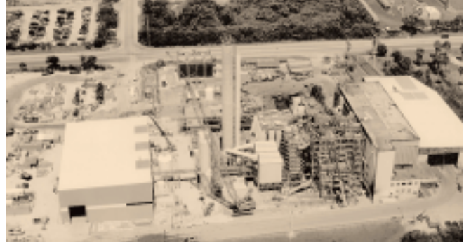
McKay Bay Refuse-to-Energy Plant Phase I completion by August, 2000 and total completion by October, 2001.
