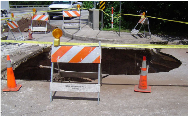
Wastewater cave-in at Sligh Avenue and Rivershore Drive.
