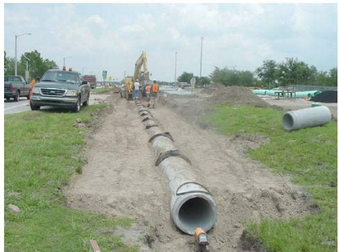
Cross Creek I - Clay Gully to Arbor Green - utility relocation prior to road construction
