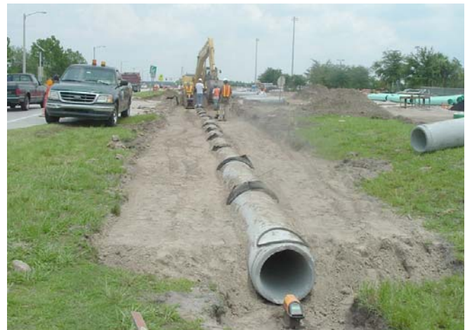
Cross Creek I - Clay Gully to Arbor Green - utility relocation prior to road construction
