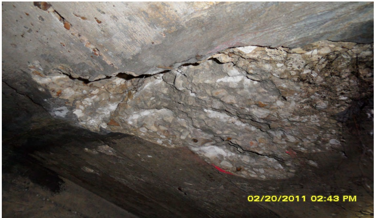
These photographs depict examples of structural problems typically found in the box culverts within the City of Tampa and are not meant to represent specific problems or locations.
