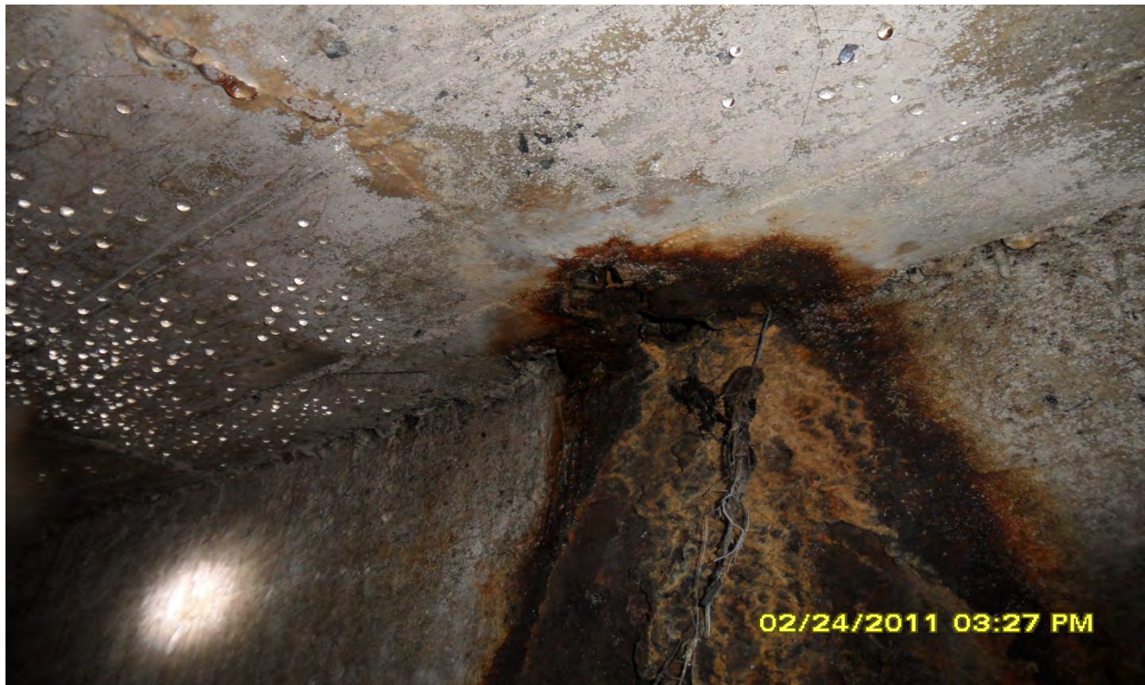
These photographs depict examples of structural problems typically found in the box culverts within the City of Tampa and are not meant to represent specific problems or locations.
