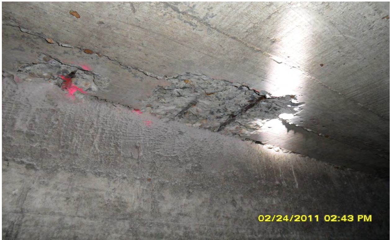
These photographs depict examples of structural problems typically found in the box culverts within the City of Tampa and are not meant to represent specific problems or locations.
