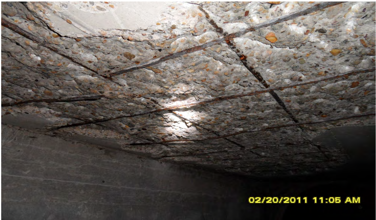
These photographs depict examples of structural problems typically found in the box culverts within the City of Tampa and are not meant to represent specific problems or locations.
