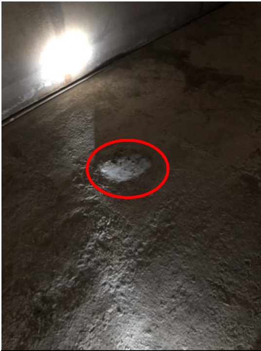
Site Picture 1 Showing A Patch on the Tank Floor Slab
