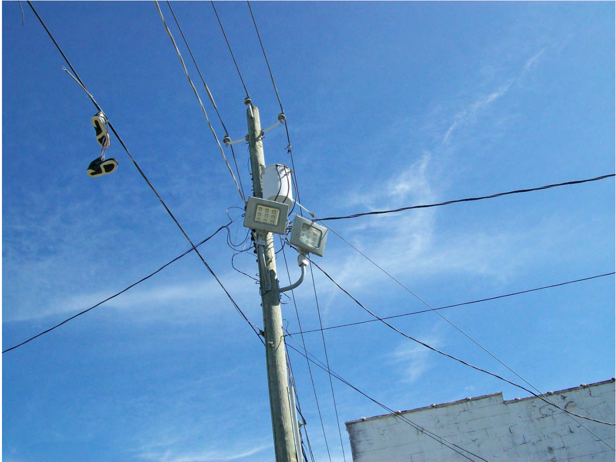
Pole Mounted Transformer
