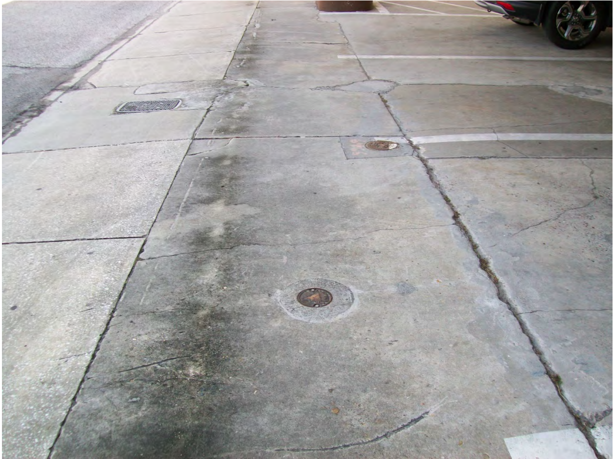
Monitoring Wells in Sidewalk
