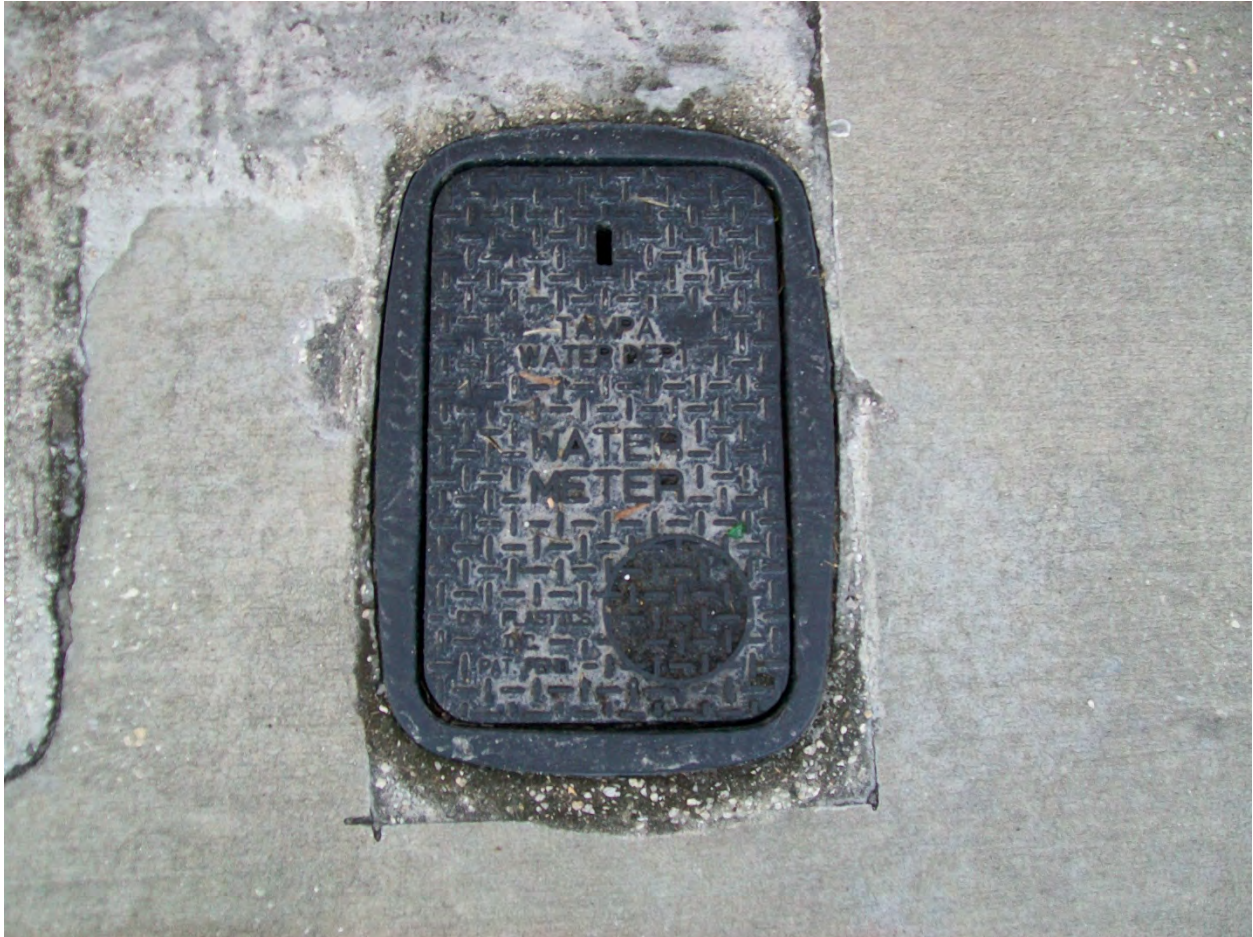
Water Meter in Sidewalk
