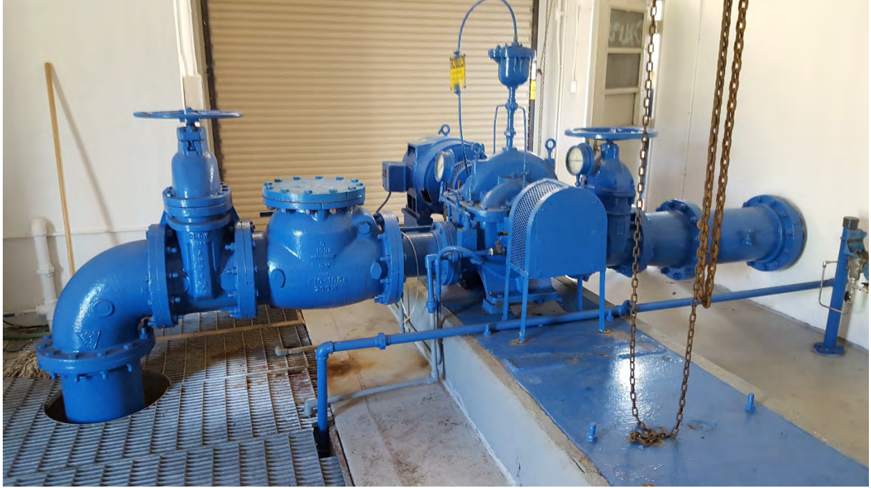
Figure 17. NWPS Piping Inside Building
