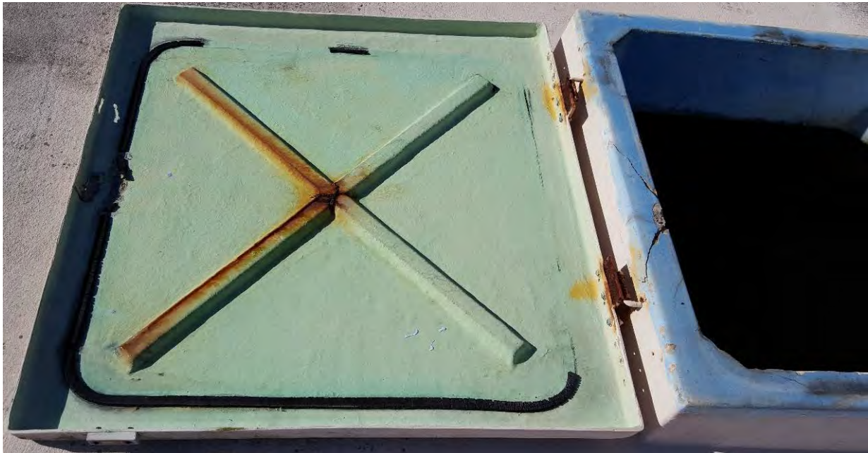
Figure 10. NWPS GST Dome Access Hatch Hardware on the fiberglass access hatch was rusting. There was cracking on the hatch curb.
