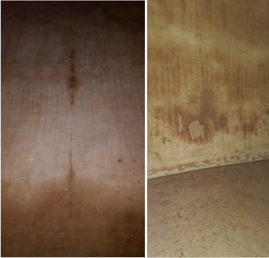
Figure 2. NWPS GST Interior Concrete Walls The interior tank wall had efflorescence along cracks in the concrete.
