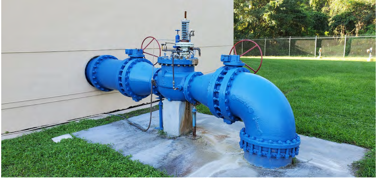
Figure 13. NWPS GST 24-inch Influent Line The altitude valve is in poor condition.
