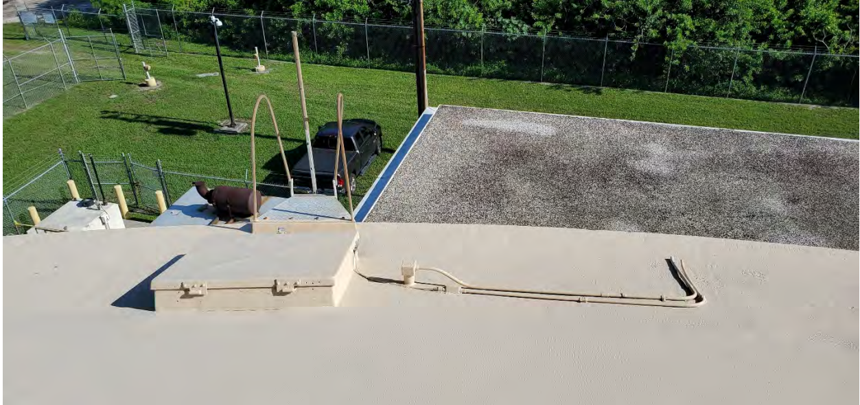
Figure 9. NWPS GST Dome Access Hatch There is no handrails and ladder cage.
