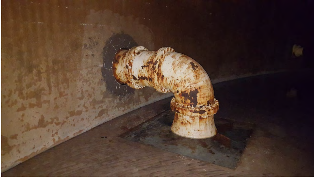
Figure 27. NWPS GST Interior DIP Pipe Corrosion on coated interior pipe.
