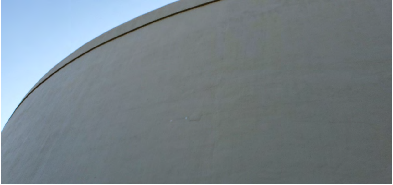
Figure 7. NWPS GST Exterior Tank Wall Cracks on the exterior tank wall.
