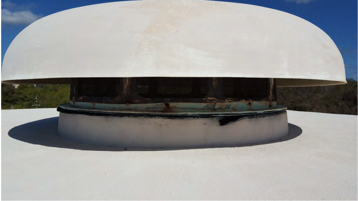
Figure 11. NWPS GST Center Dome Vent Corrosion on metal vent supports and cracking on vent curb.
