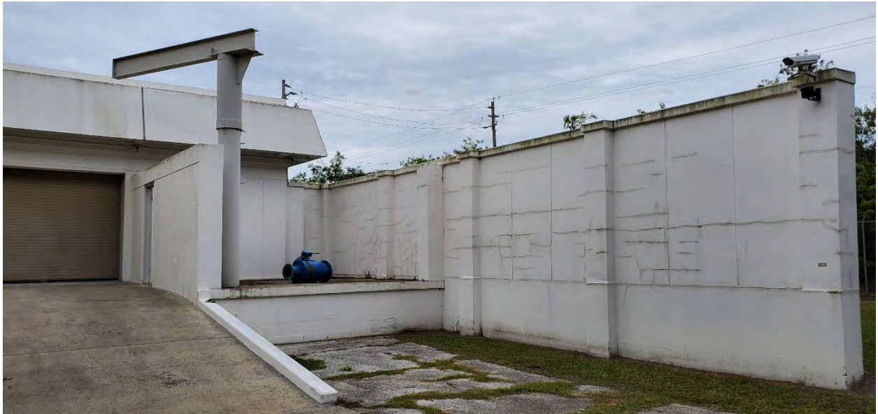
Figure 16. NWPS Building Exterior The wall is in poor condition.
