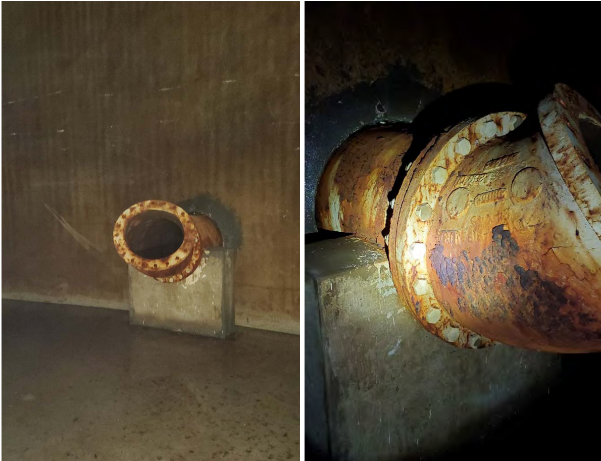
Figure 4. NWPS GST Interior DIP Pipe Corrosion on coated interior pipe.
