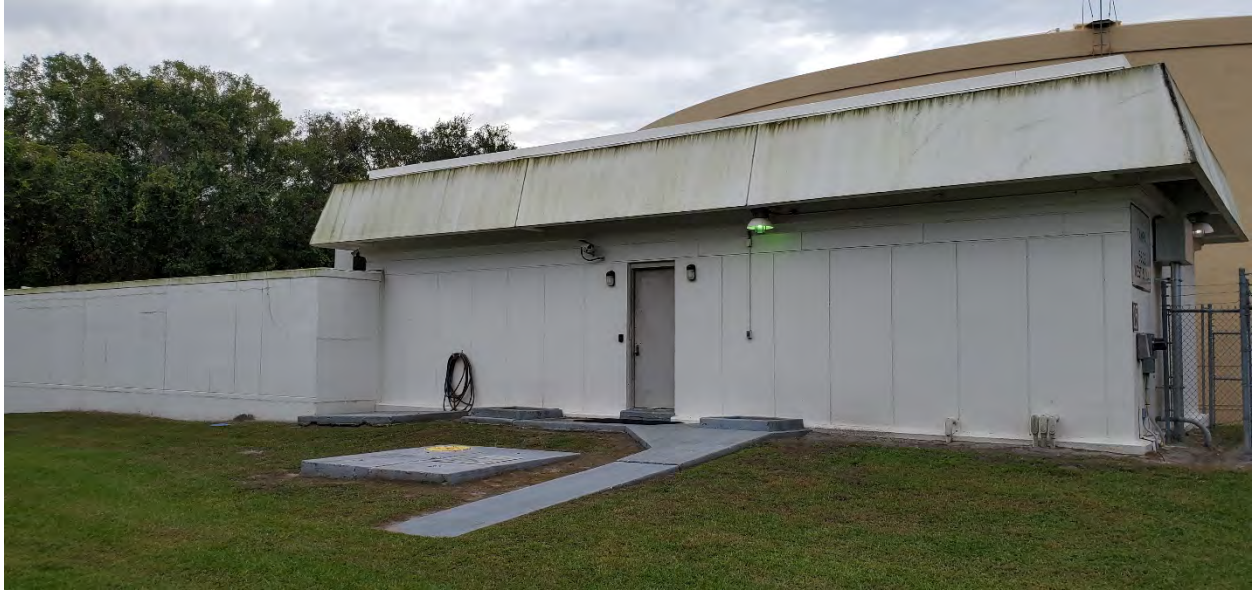
Figure 15. NWPS Building Exterior The wall is in poor condition.
