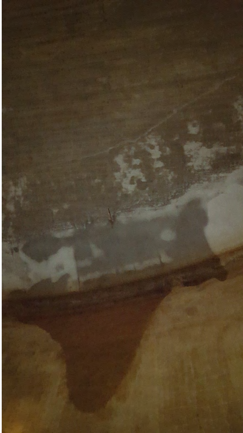
Figure 3. NWPS GST Interior Dome Cracks were present in the tank interior dome.
