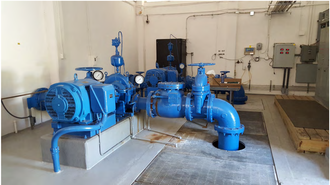
Figure 18. NWPS Piping Inside Building
