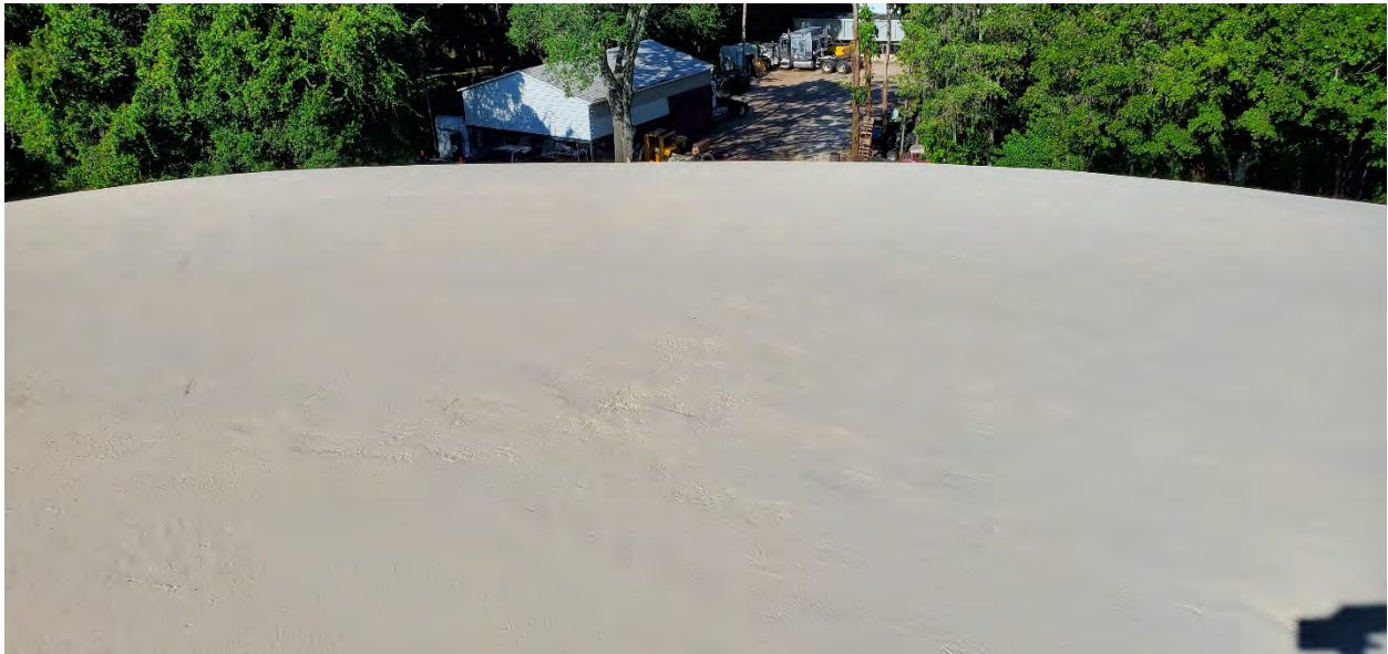
Figure 12. NWPS GST Dome Cracks were not visible on the dome.
