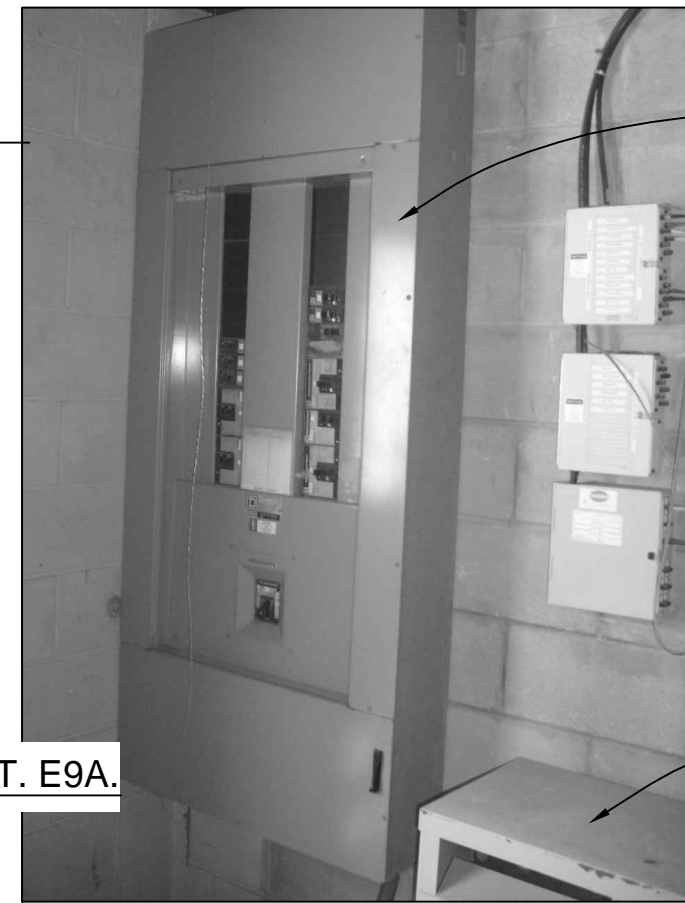
PANELBOARD CARPENTER SHOP ELECTRICAL ROOM TRANSFORMER
