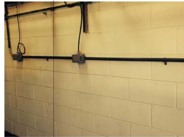
PHOTO No.1 (EVAPORATOR ROOM)
