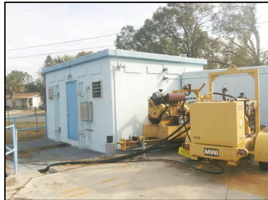
POINSETTIA AVENUE STORMWATER PUMP STATION
