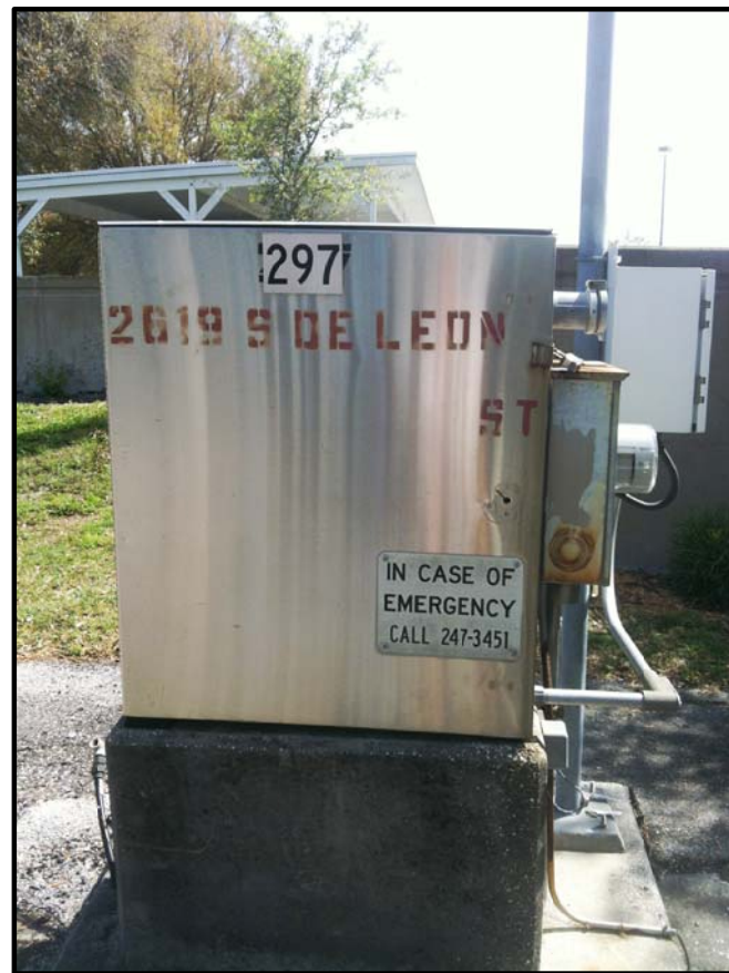
AMI HOSPITAL STORMWATER PUMP STATION
