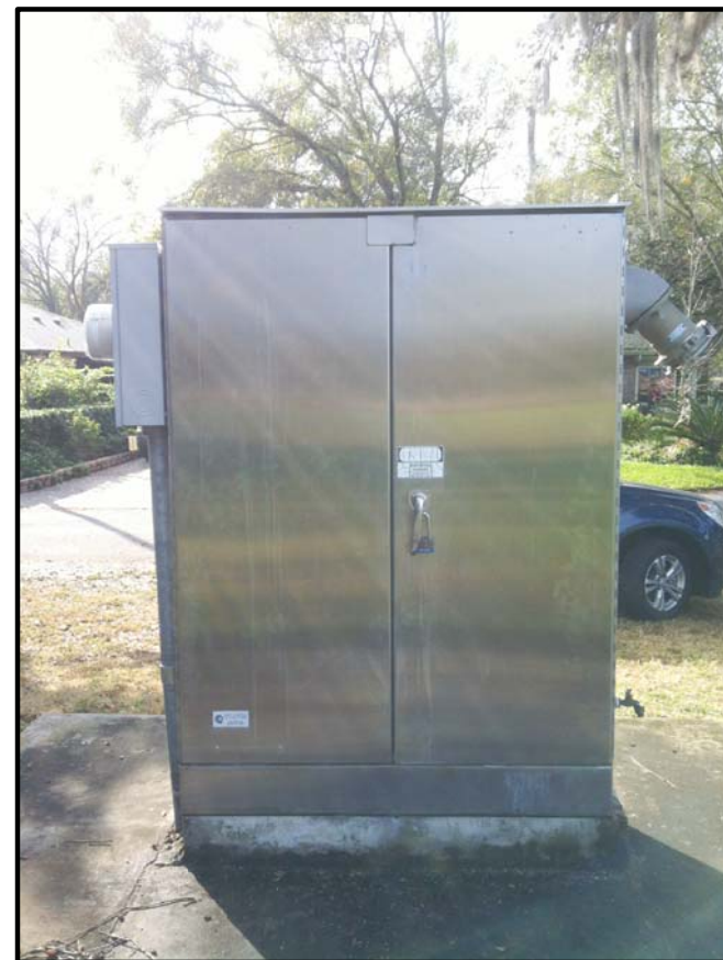
PENALTY LAKE STORMWATER PUMP STATION
