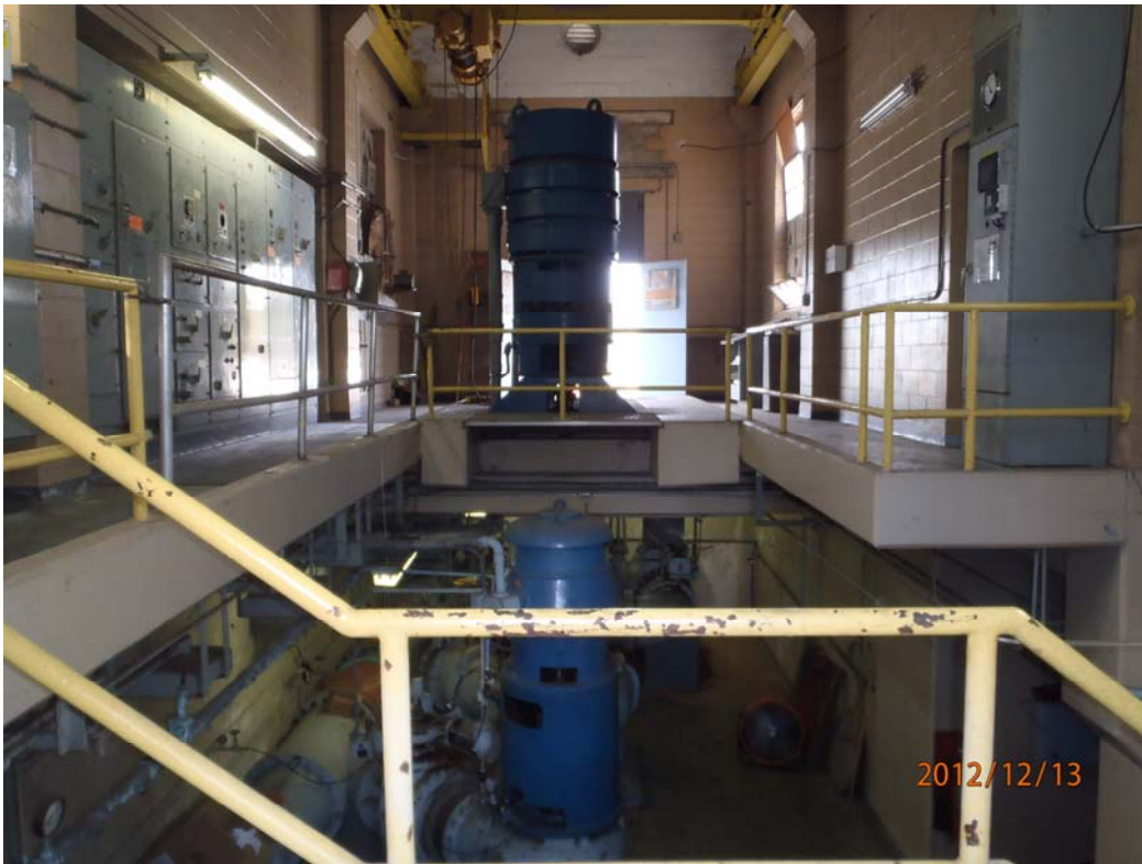
Photograph 2- General view of pump motors and inside of building.
