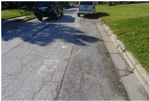
Cracking and Patching At 3123 W. Kensington Ave
