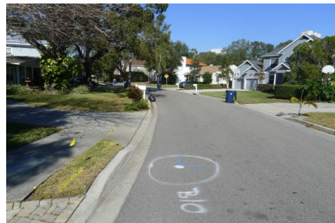
Good Pavement Condition at South End Of Waverly Place [Asphalt Thickness = 10 inches]
