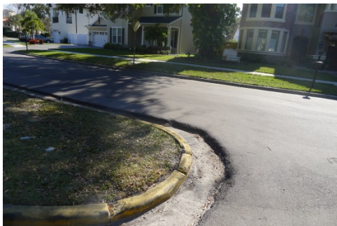
Excessive Overlay For South "Y" At East End of W. Kensington Avenue
