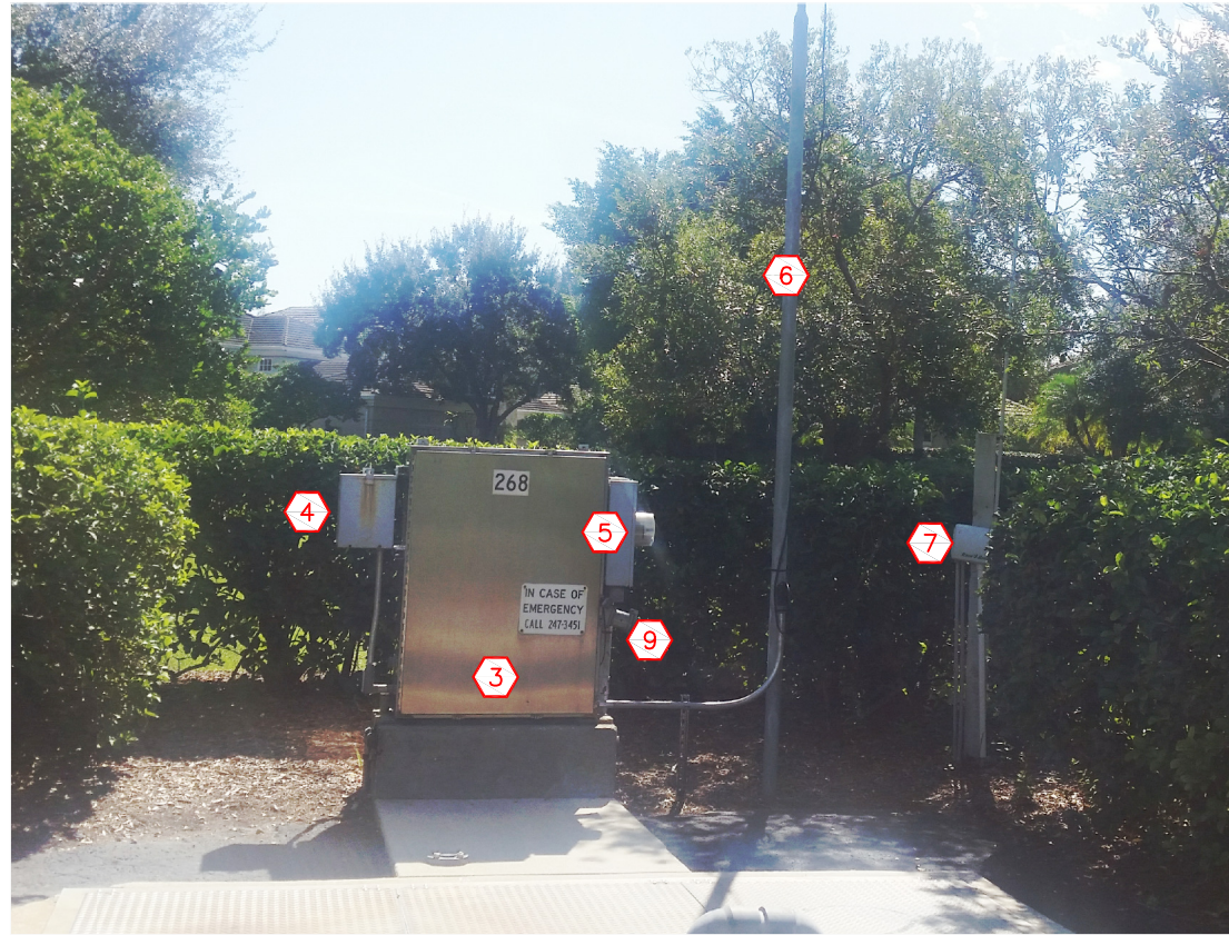
EX. CONTROL PANEL SOUTH VIEW
