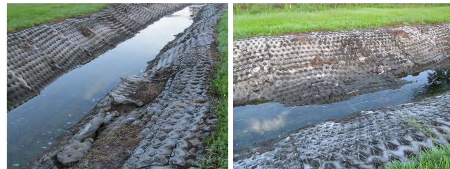
Flow Under Mat Displaced and Broke Mat
