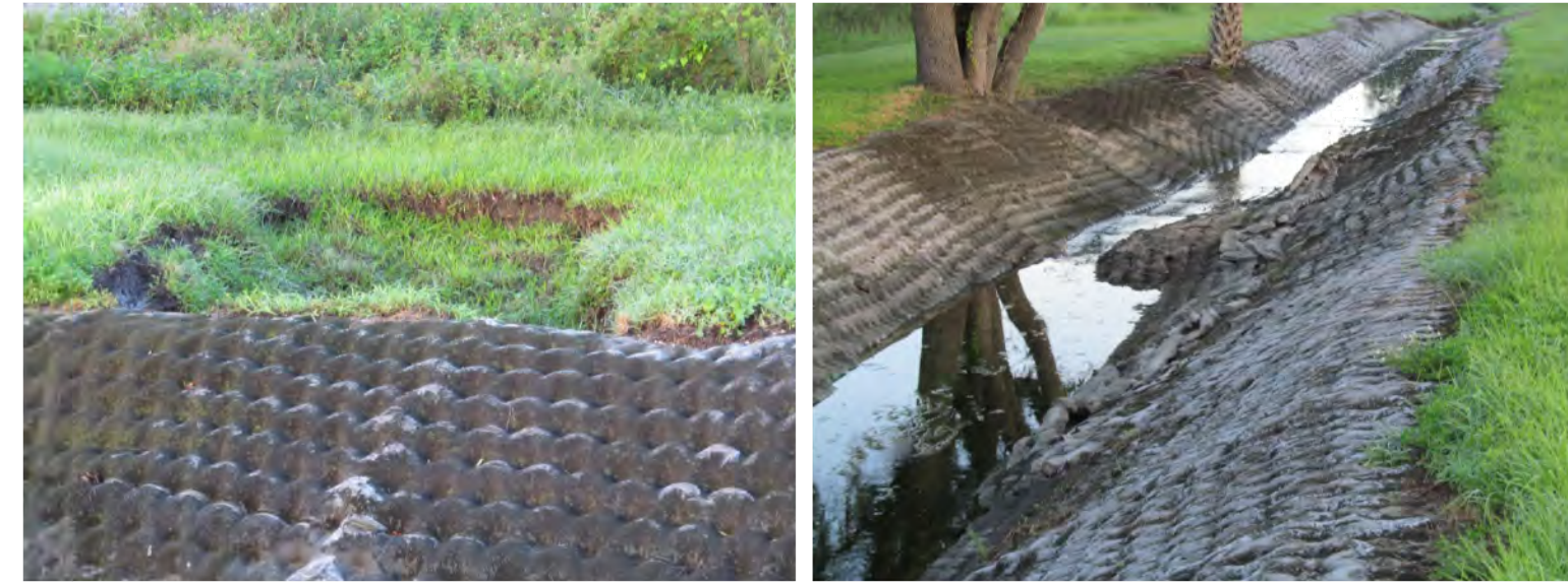
Overflow Caused Erosion Under the Concrete Mat
