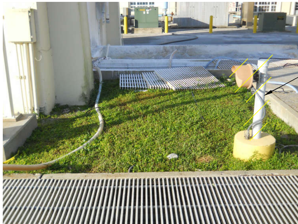
RELOCATION OF MICROWAVE SIGNAL TRANSMITTER – VIEW 1
