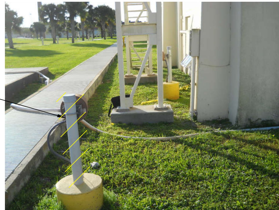
RELOCATION OF MICROWAVE SIGNAL TRANSMITTER – VIEW 2
