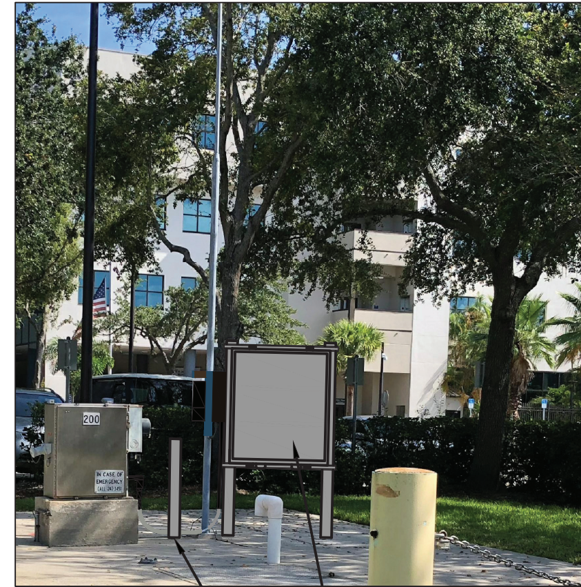
PROPOSED CONDUIT SUPPORT TUBE COLUMN (SEE ELECTRICAL SHEETS) PROPOSED PUMP CONTROL PANEL (SEE ELECTRICAL SHEET E1 FOR PROPOSED EQUIPMENT LAYOUT)
