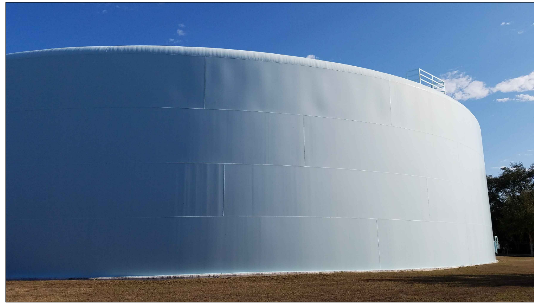
Figure 2 - All exterior surfaces exhibiting paint peeling shall be cleaned and re-coated as specified.
