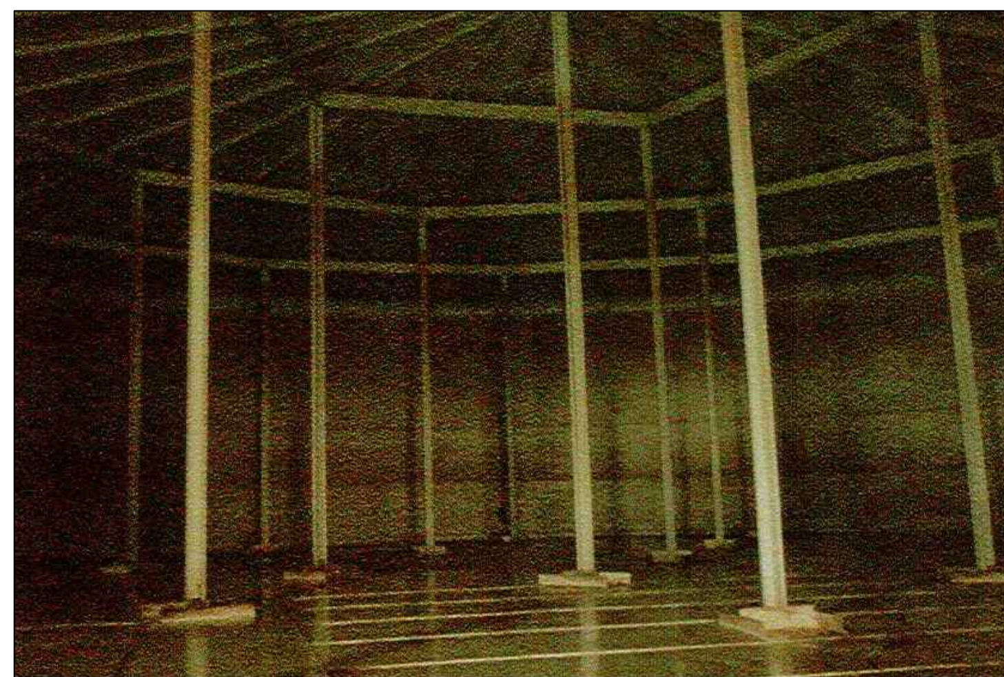
Figure 8 - All rafter surfaces exhibiting rust shall be cleaned and re-coated as specified.
