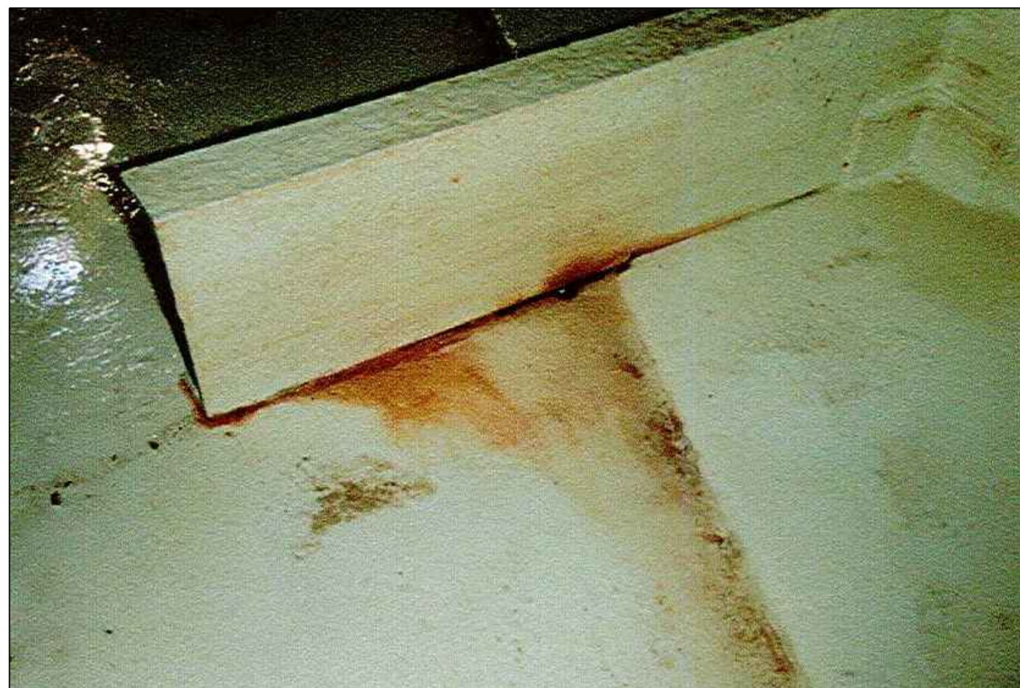
Figure 5 - All floor surfaces exhibiting rust shall be cleaned and re-coated as specified.
