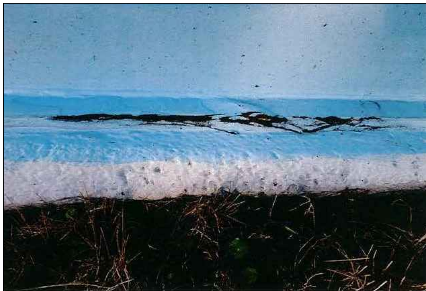
Figure 4 - All exterior chime surfaces exhibiting rust shall be cleaned and re-coated as specified.
