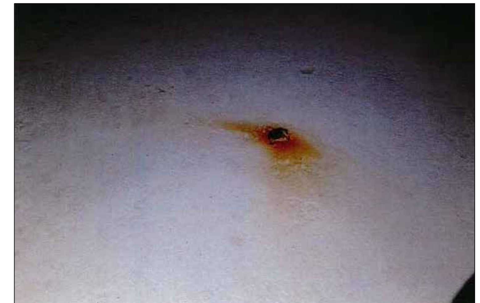
Figure 6 - All floor surfaces exhibiting rust shall be cleaned and re-coated as specified.
