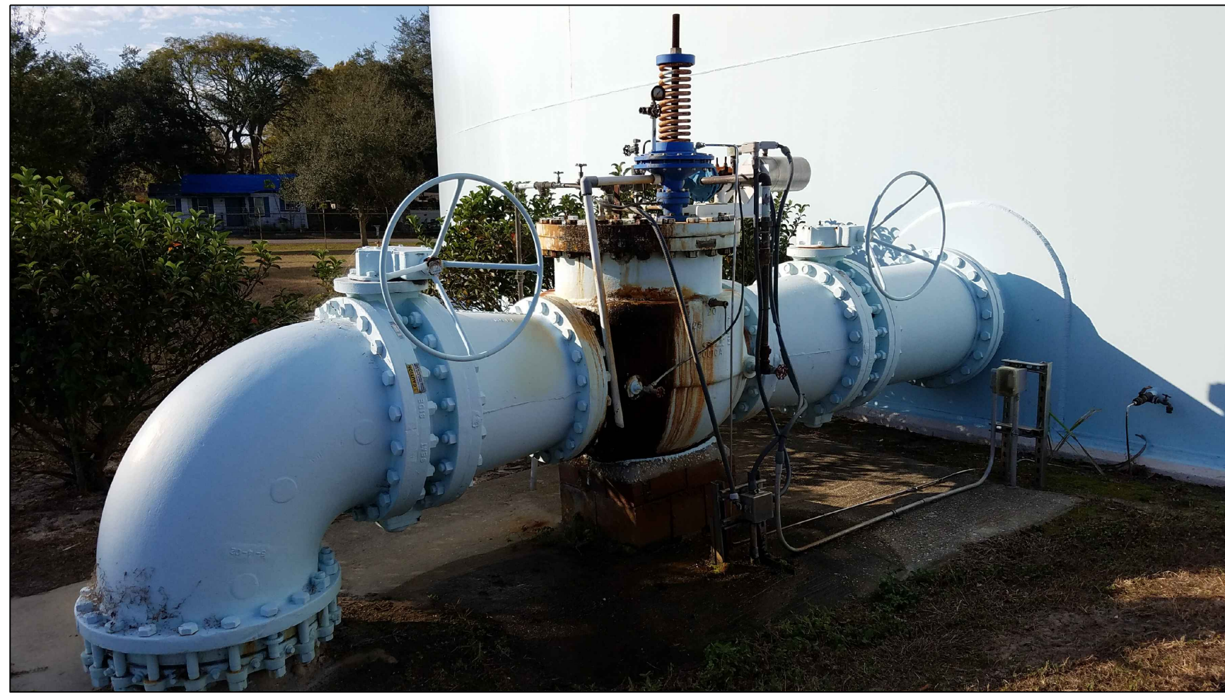
Figure 1 - Remove and replace existing altitude valve and piping as specified. New valves, piping and fittings shall be factory and field coated as specified.
