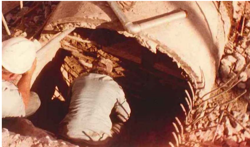
Photograph 10 – Cut Pipe (note double row of steel reinforcing), March 24, 1984, Harbour Island Relocation
