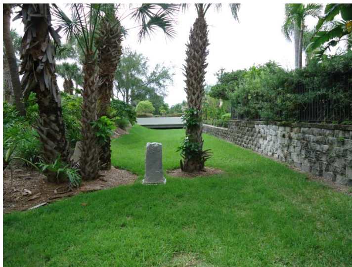
Photograph 11 – Air Release Valve with Fake Rock Enclosure, note Low Bridge Beyond
