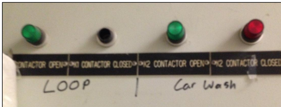
PHOTO 6 CONTACTOR BULBS BURNT OUT
