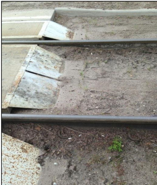
PHOTO 25 RAIL WITHOUT INSULATING BOOT
