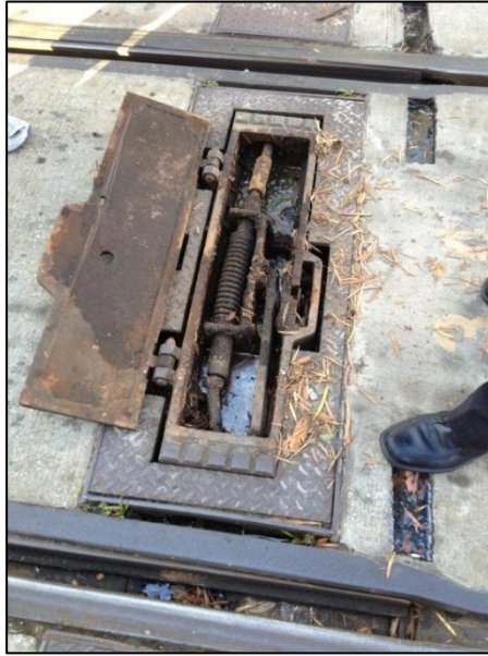
PHOTO 1 OLD SWITCH MACHINE
