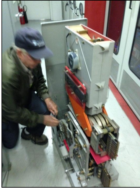
PHOTO 16 FEEDER #1 RACKED TO INSPECT CAUSE OF FAILURE
