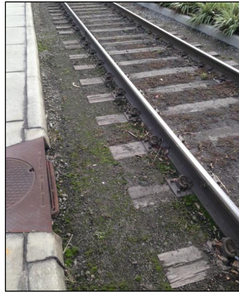
PHOTO 26 TRACKS WITHOUT RAIL BOOT INSULATION
