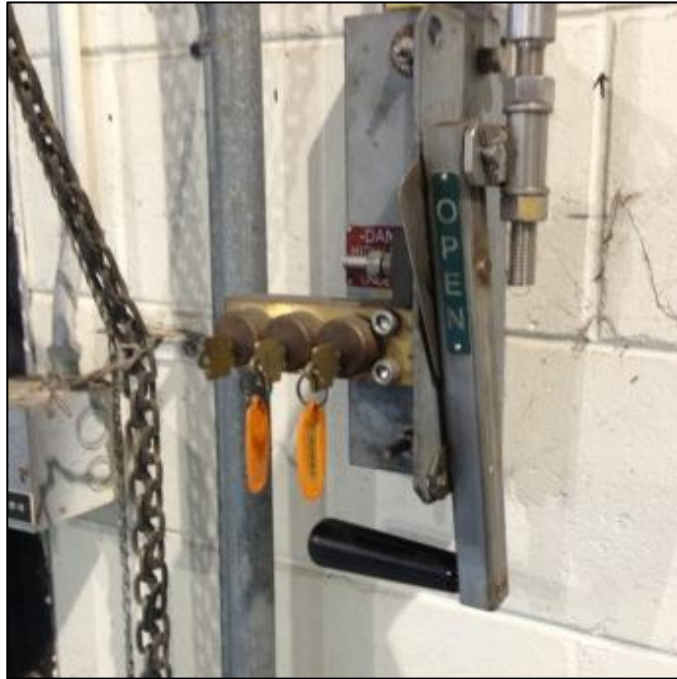
PHOTO 13 KEY INTERLOCK AT CATENARY SWITCH
