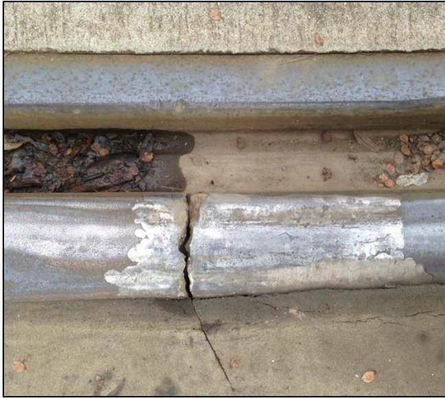
PHOTO 22 BROKEN RAIL WELD AT 17 TH STREET AND 8 TH AVENUE
