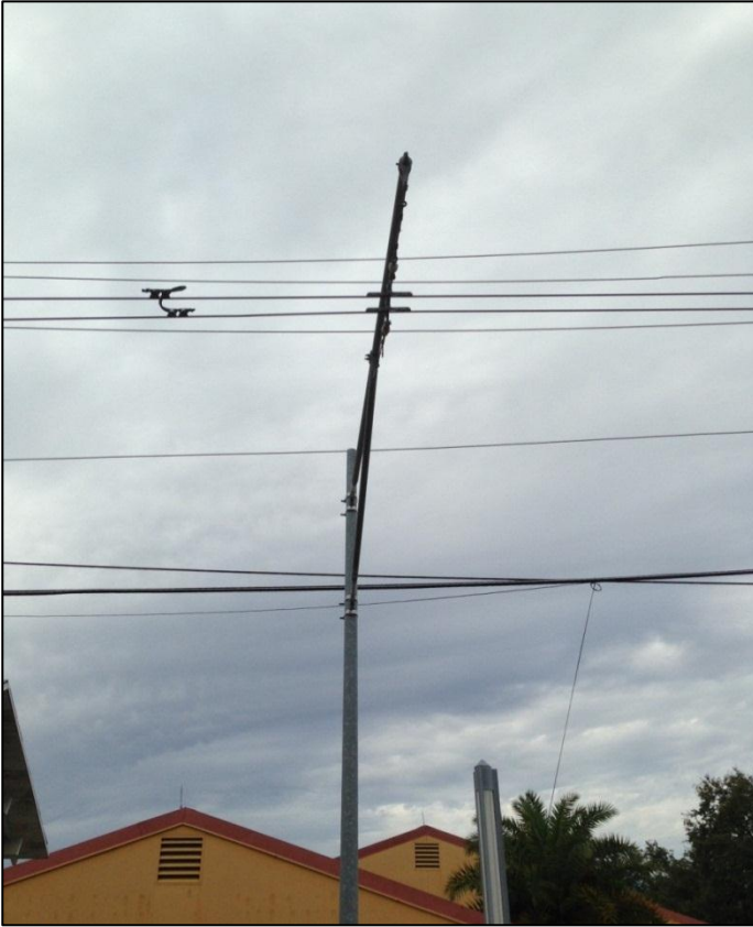
PHOTO 20 CANTILEVER ARM SHOWN NOT PERPENDICULAR TO THE TRACK NORTH OF CADRECHA PLAZA STATION
