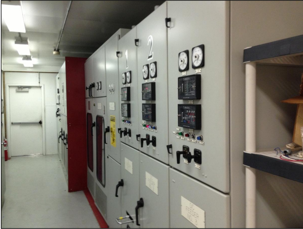
PHOTO 19 SOUTH TRACTION POWER SUBSTATION
