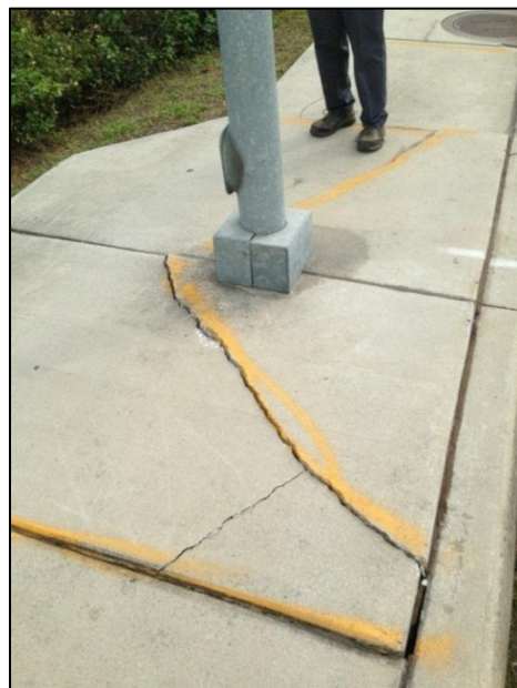
PHOTO 29 SIDEWALK DAMAGE DUE TO FLOODING AT TRACK LEVEL
