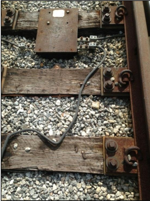
PHOTO 27 NEUTRAL RETURN CABLES AT CSX CROSSING
