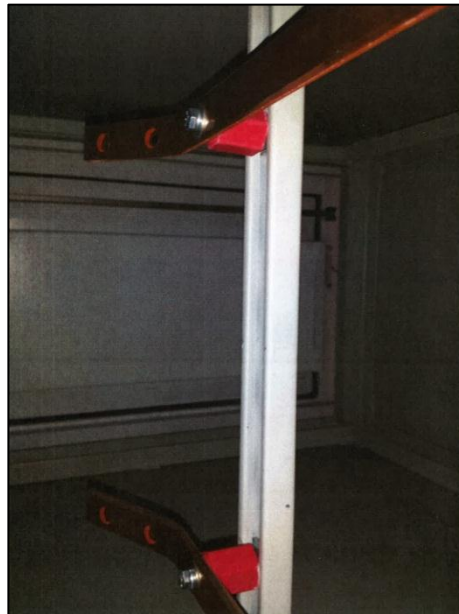
PHOTO 18 FNAG SWITCH WITH NO CONNECTING CABLES
