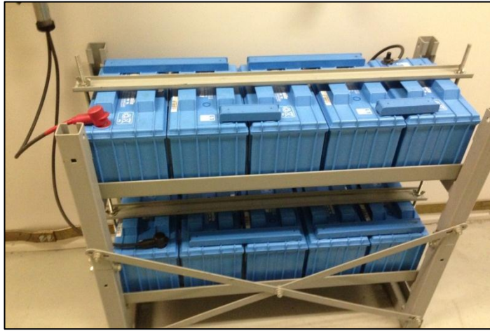
PHOTO 14 CONTROL POWER BATTERIES
