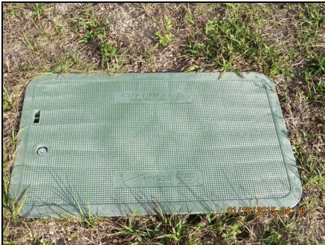
Verizon underground utilities on the east side of 46 th Street north of Whiteway Drive.
