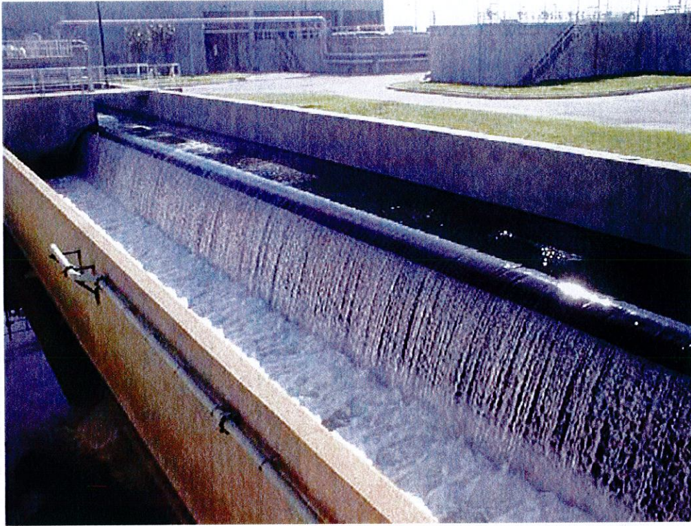
Figure 4-2 Aeration occurring at Post Aeration Chlorination Tanks
