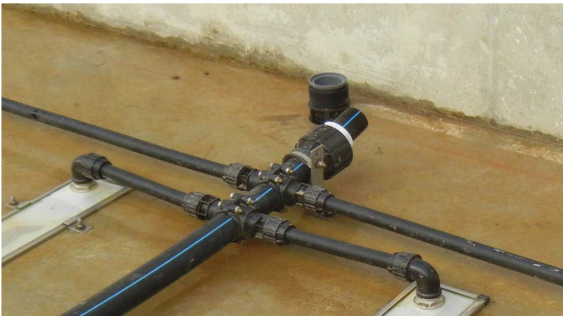
HDPE Drop and Connections
