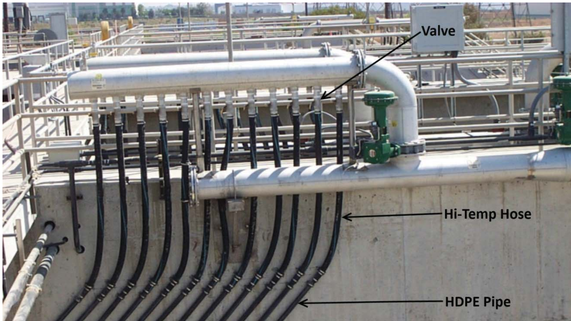
HDPE Drop-Pipes on Individual Valves
