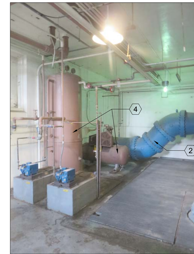
VIEW OF AREA OF CONDENSING ROOM 3 DEPICTING PIPE ROUTING AND COMPRESSOR AND TANKS.
