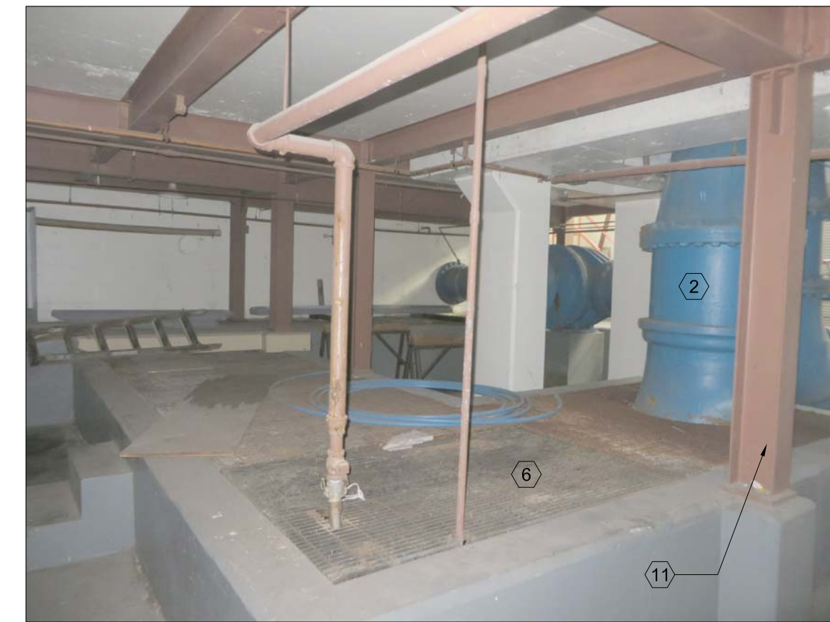
VIEW OF AREA OF CONDENSING ROOM 1 DEPICTING PIPE ROUTING AND COMPRESSOR AND STRUCTURAL STEEL FRAMING.
