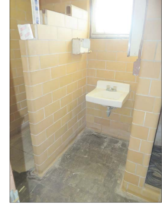
VIEW OF EXISTING TOILET ROOM SHOWING EXISTING PLUMBING FIXTURES AND GLAZED MASONRY UNITS TO BE CLEANED AND REPAIRED. FLOOR FINISH TO BE REPLACED.
