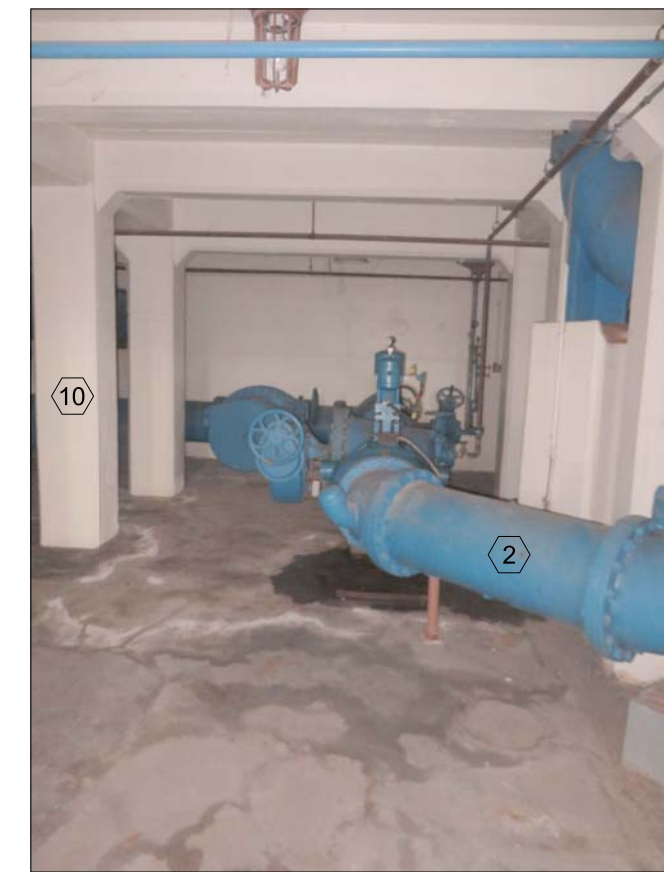
VIEW OF AREA OF CONDENSING ROOM 2 DEPICTING PIPE ROUTING.
