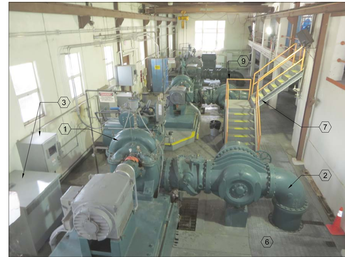
VIEW LOOKING DOWN TO THE LOW LIFT PUMP ROOM
