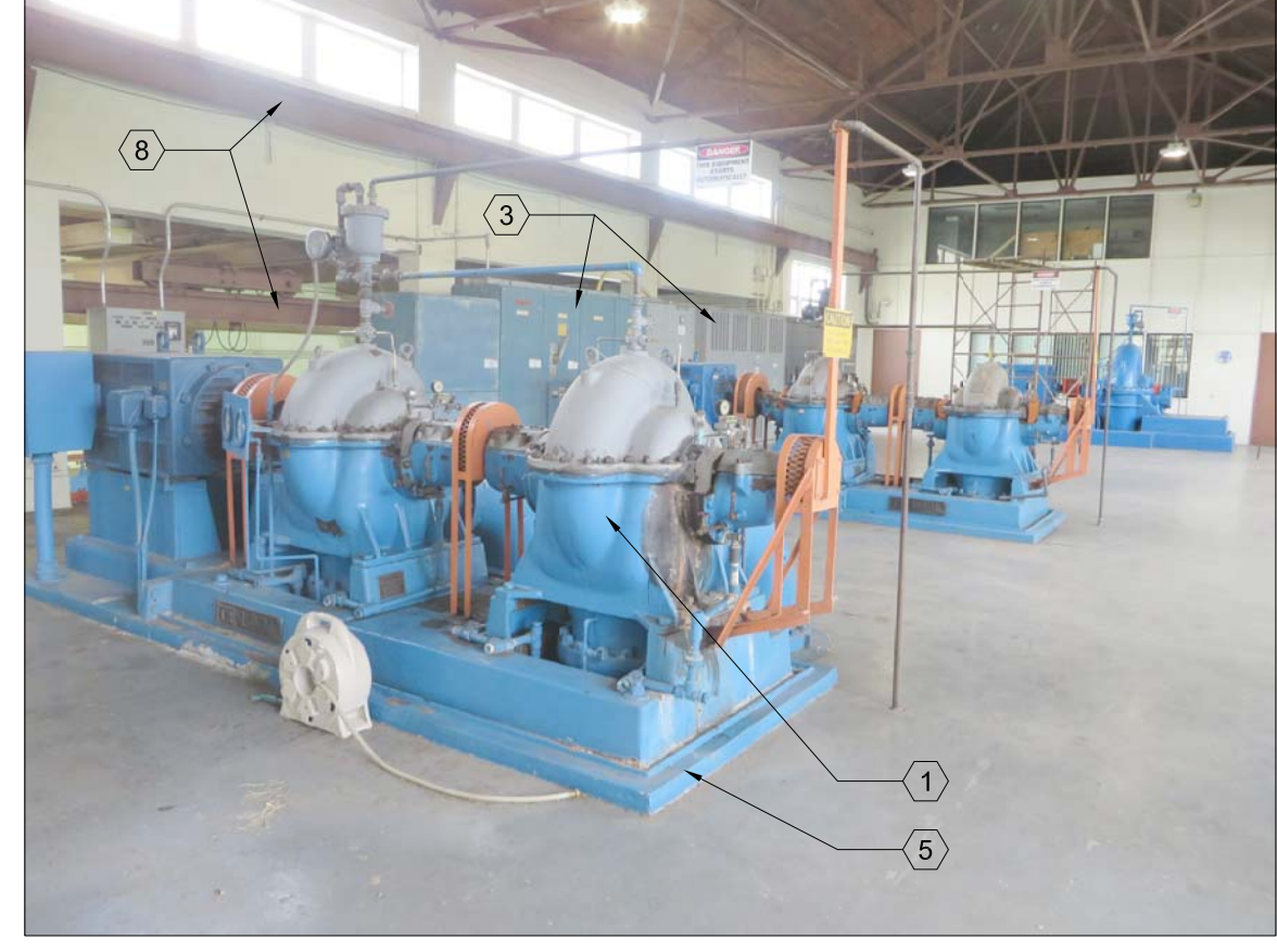
VIEW OF HIGH LIFT PUMP ROOM SHOWING PUMPING MACHINERY AND ELECTRICAL EQUIPMENT
