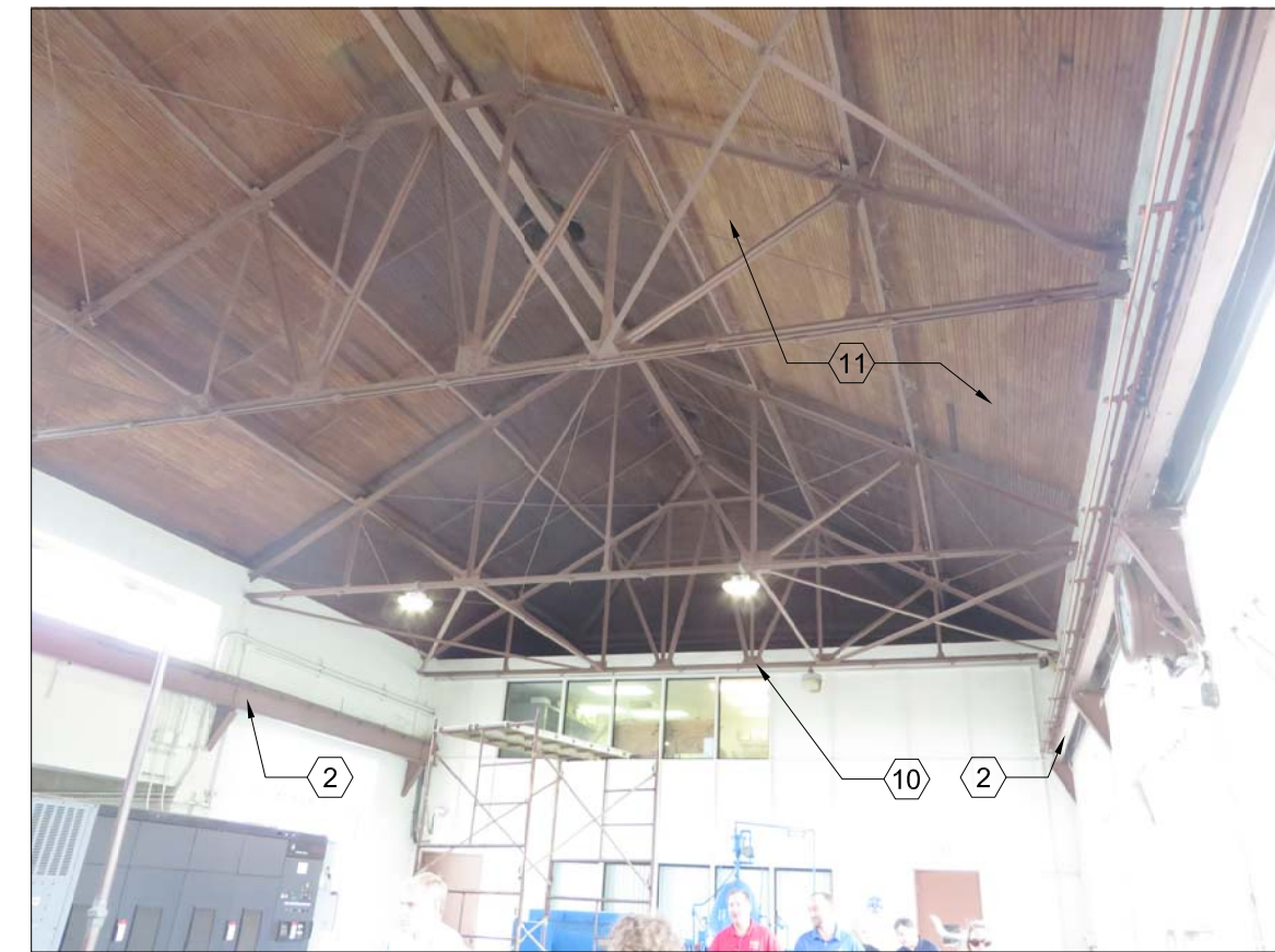
VIEW OF CRANE RAILS, STRUCTURAL STEEL TRUSS FRAMING, ROOF DECKING, LIGHT FIXTURES, CLERESTORY WINDOWS.
