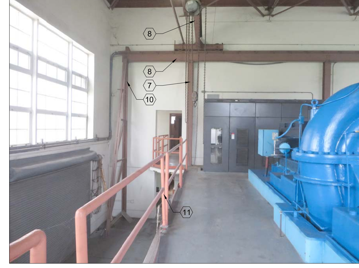
VIEW OF THE END OF THE HIGH LIFT PUMP ROOM SHOWING PUMPING MACHINERY, ELECTRICAL EQUIPMENT (TO BE ADJUSTED TO PROVIDE ACCESS TO TOILET AND LOCKER ROOMS), STEEL COLUMNS, CRANE RAIL, AND CRANE BEAM.
