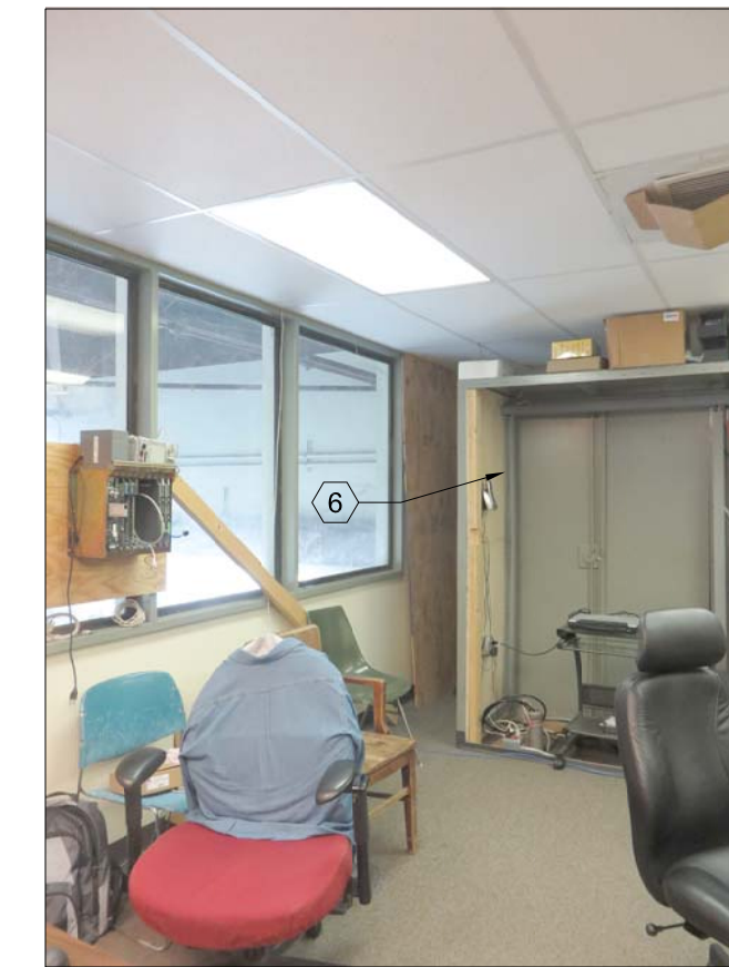
VIEW OF I & C DEVELOPMENT ROOM DEPICTING CABINETS TO BE REMOVED, EXISTING FINISHES TO BE REPLACED.
