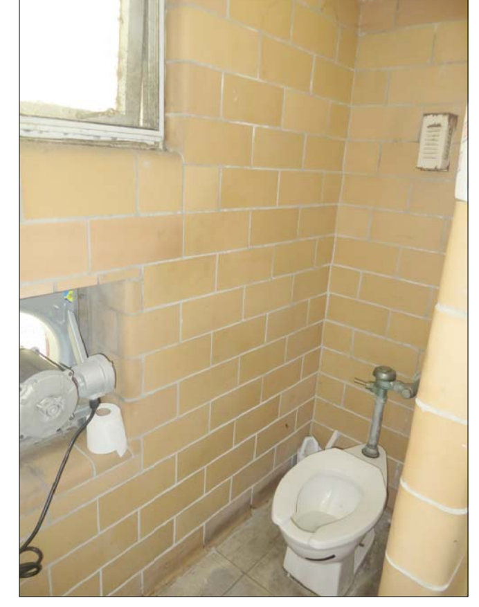
VIEW OF EXISTING TOILET ROOM SHOWING EXISTING PLUMBING FIXTURES AND GLAZED MASONRY UNITS TO BE CLEANED AND REPAIRED. FLOOR FINISH TO BE REPLACED. WALL MOUNTED EXHAUST FAN TO BE REMOVED.
